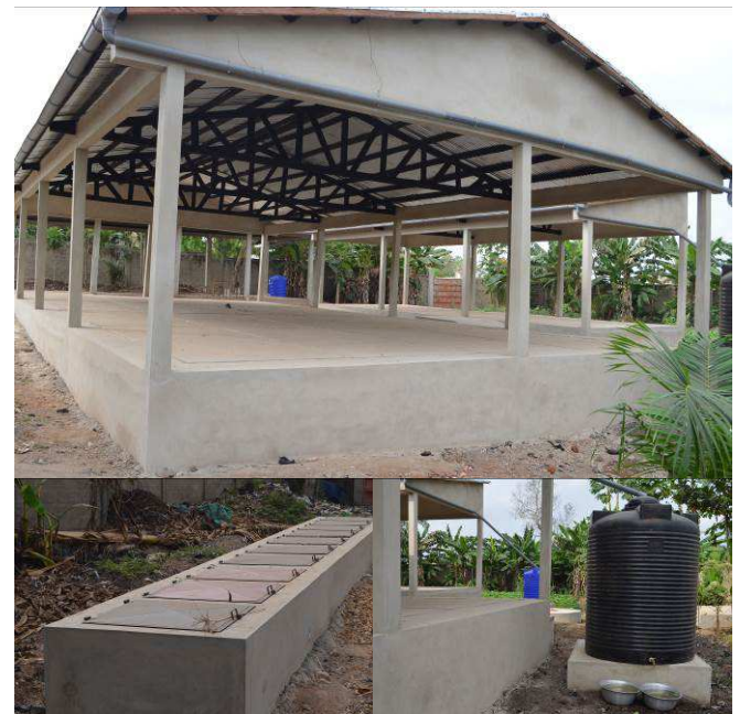
Fig. 10: Sheds, drying beds and rain water harvesting system of the composting plant of Lokossa (source: E. Albert, 2014)
