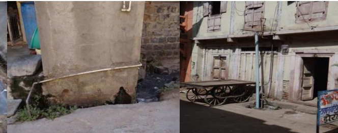
Some places septic tanks are below the toilets
