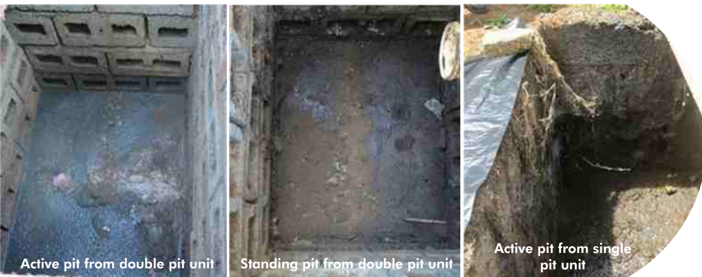
Fig.10. Photographs of pits from hand pouring low flush units.
