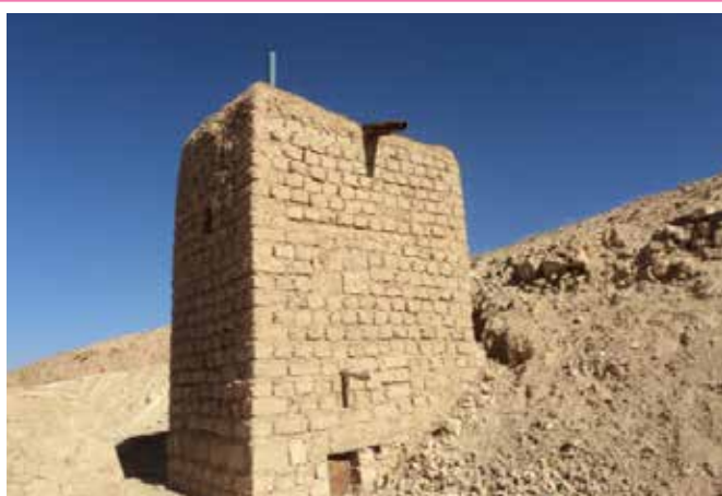
Raised urine diversion pit latrine with urine pipe exit exposed to the atmosphere, Afghanistan (Photo: ACF, Afghanistan)
