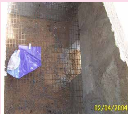
Fire grill inside incinerator
