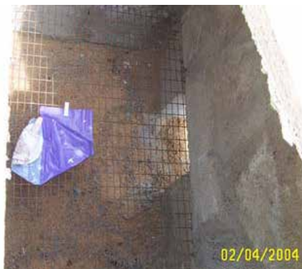
Fire grill inside incinerator
