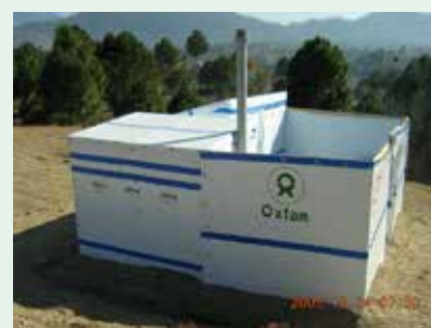
Screened latrine and bathing unit
