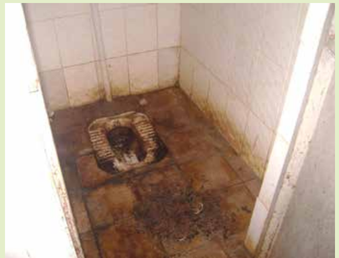
Poor maintenance and cleanliness can lead to girls not using latrines
