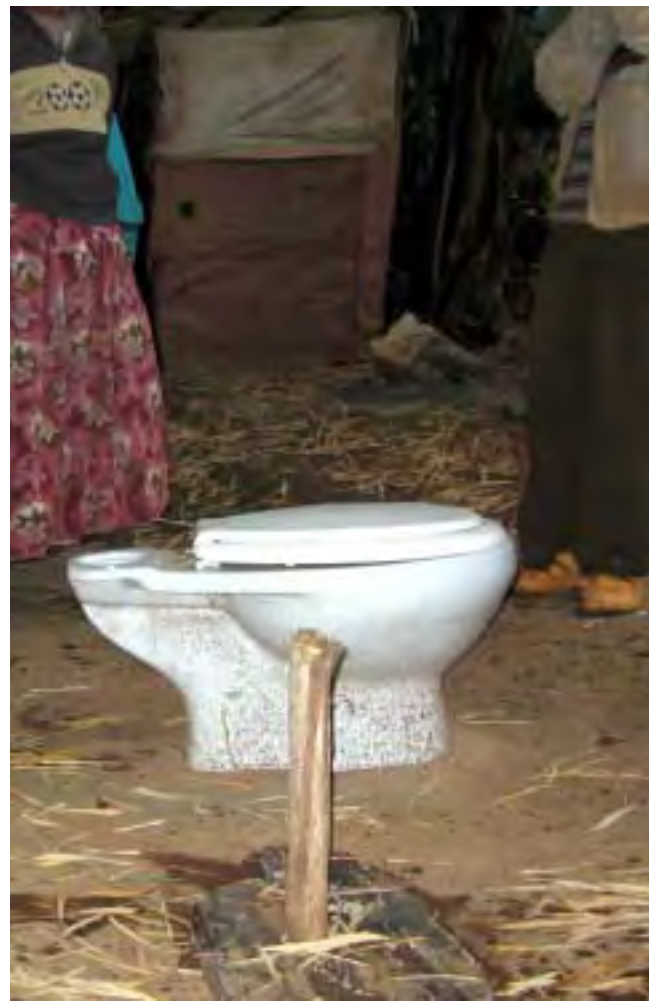
ABOVE After achievement of ODF status, the standard and quality of latrines tends to improve gradually. Households find reasons to invest and improve the quality of toilets from the initial low cost pit latrines they constructed after triggering. A villager who runs a backpackers tourist camp in Chench Woreda, Goma Gofa zone in southern Ethiopia understood the need for providing toilet facilities for tourists. In the background, a makeshift latrine constructed immediately after triggering of CLTS is visible.
