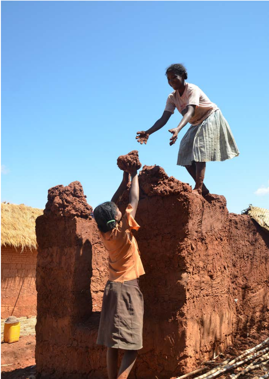
Zinah and her daughter, Zin, 13 years old, building their toilet. Ambohimasina village, Talatan' Angavo commune, Ankazobe district, Analamanga region, Madagascar. October 2013. Credit: WaterAid/ Ernest Randriamalala.
