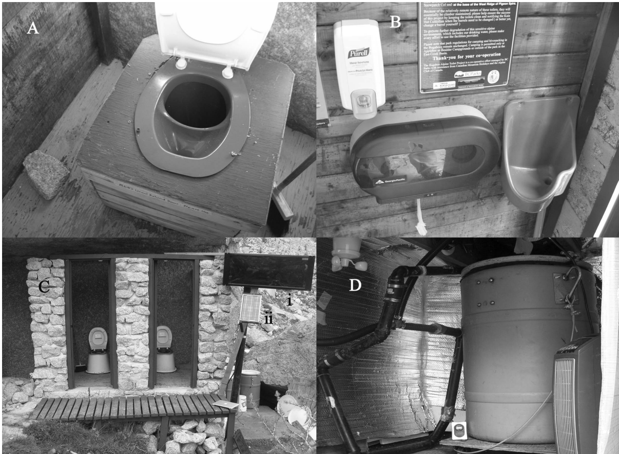
Fig. 2.1 Alternative toilet waste management treatments at Kain Hut, Bugaboo Park, B.C. Canada. A) Urine diversion toilet seat. B) Urinal with 1” braided drain pipe to collection barrel. C) Lower toilets with UD12V solar hot air panel (i) above a 5W PV panel (ii). D) Upper Kain Hut toilet insulated basement, 110V heater, and 110CFM exhaust fan positioned around a 200L plastic barrel with double garbage bags to collect solids.
