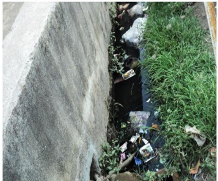
Widespread clogging of drains
