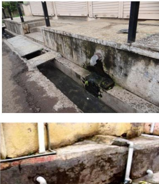
Effluent and grey-water being discharged into drains
