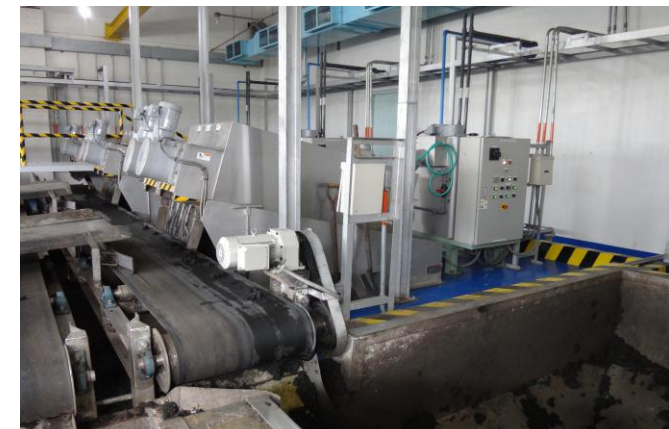
Sludge treatment for reuse
