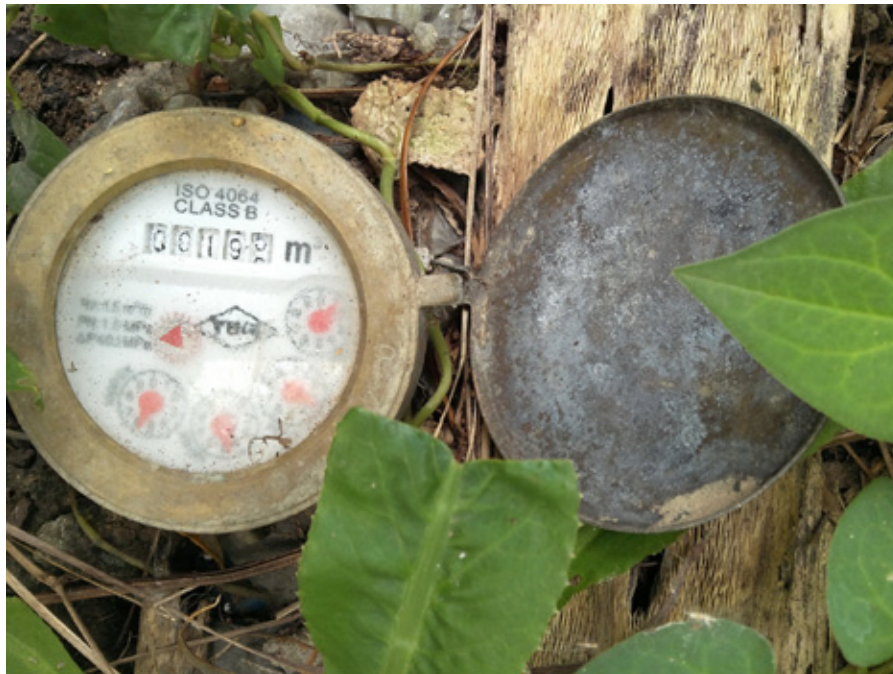
FIGURE 5 WATER METER AT HOUSEHOLD SERVED BY SMALL WATER ENTERPRISE IN MEKONG
