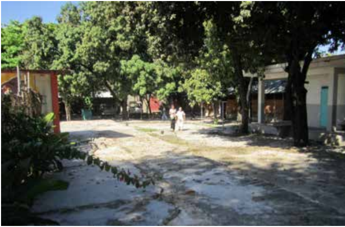
Figure 13: 100m of biogas pipe was laid across a school in Tabarre, but never used (TF 020).
