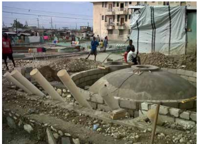
Photo VR_10: biodigester LaSaline, Sloped inlet pipes off to the side.
