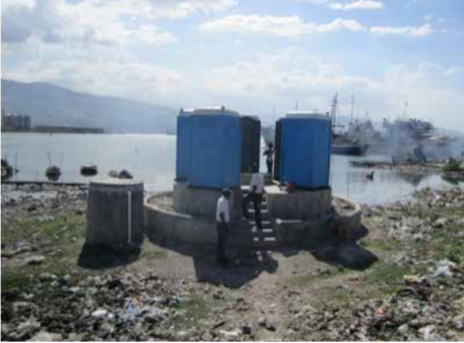
Photo VR_7: Emergency biodigester in Wharf Jeremy.
