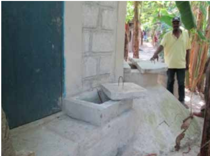
Photo ADR_1: Household biodigester showing portal for animal waste.
