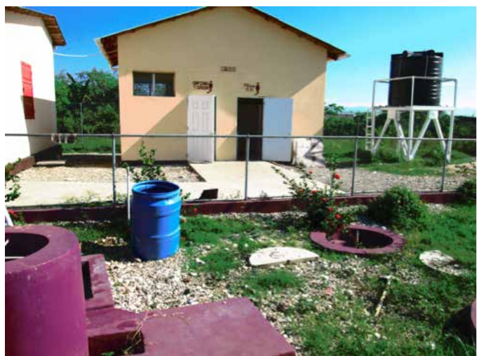
Figure 4 Biodigester at 'Ecole ASPAM' (TF 115) showing biodigester and animal waste port in foreground, toilet block in middle ground, and water supply in background. Making all of these elements work in unison, was unachievable in most cases.
