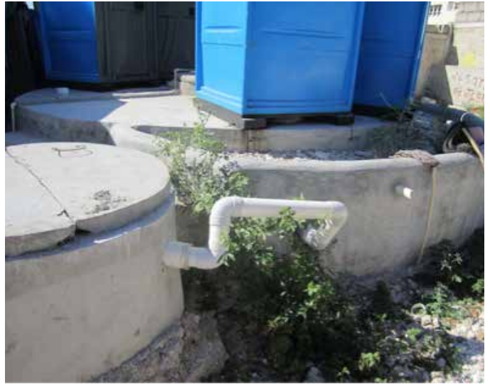
Figure 10: Simple plumbing requirements of biodigesters were often misunderstood.
