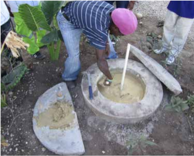
Figure 9: Details like finishing the top of a biodigester with clay rather than cement, were overlooked.
