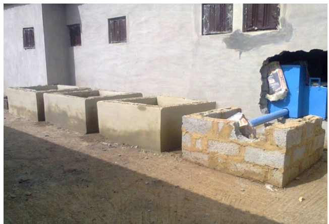
Primary treatment pit
