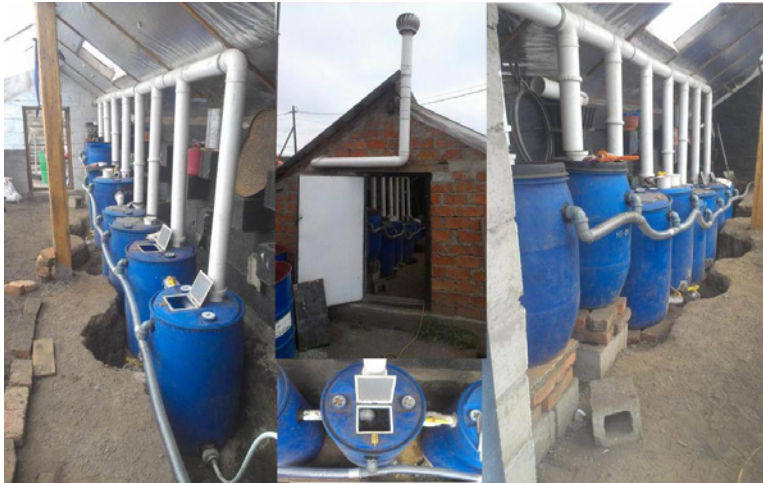
Figure 3 Flow Diagram (above) and photo (below) of Greenhouse Greywater Treatment Unit (Photo Credit to S.M.N. Uddin, July 2013)
