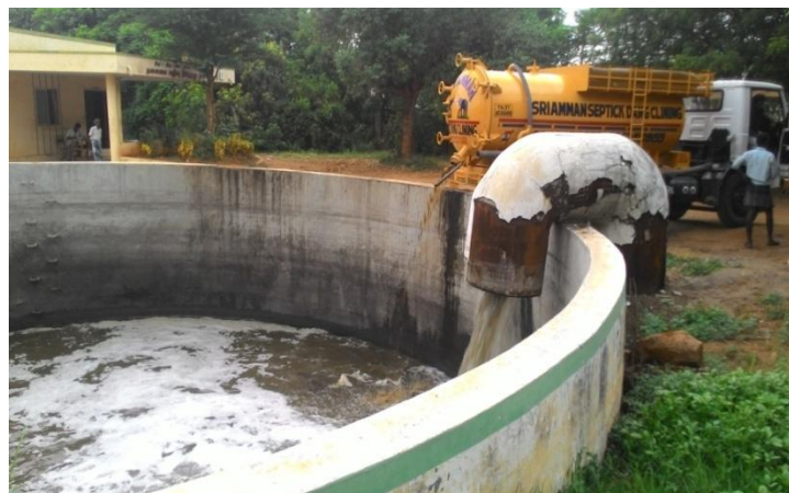
Figure 4: Septic tank connected to community toilet in Ariamangalam slum (Source: Bhitush/CSE, 2015)
