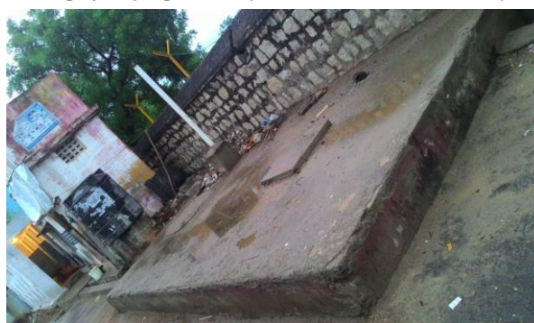
Figure 2: Septic tank connected to community toilet in Ariamangalam slum (Source: Bhitush/CSE, 2015)
