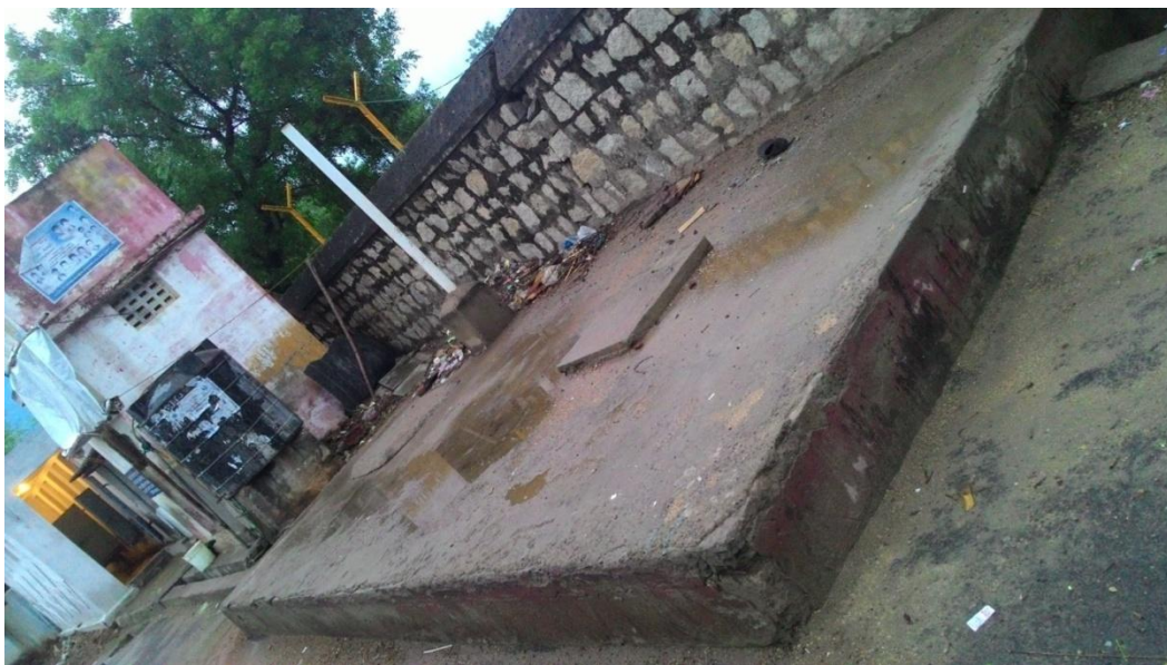
Figure 2: Septic tank connected to community toilet in Ariamangalam slum (Source: Bhitush/CSE, 2015)
