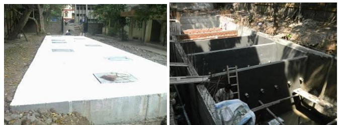
Fig. 9: Anaerobic treatment in COEP hostel (source: ESF; 2015)
