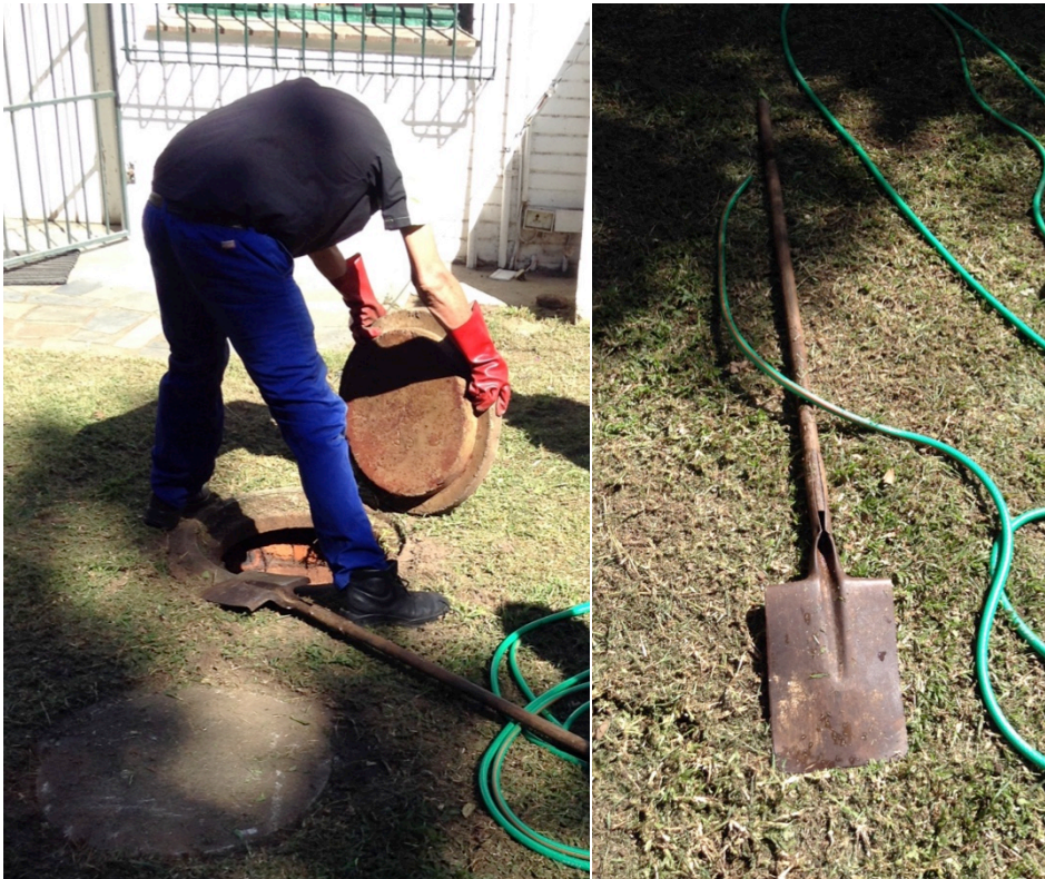
Figure 15: Opening the first compartment of the septic tank and the equipment used
