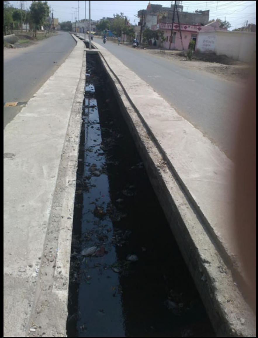
Open drain in the middle of the road, but referred as sewer line, Dewas, MP
