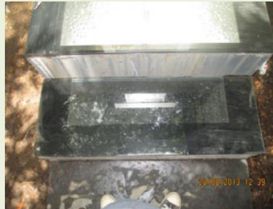
Glass window to monitor solids pit
