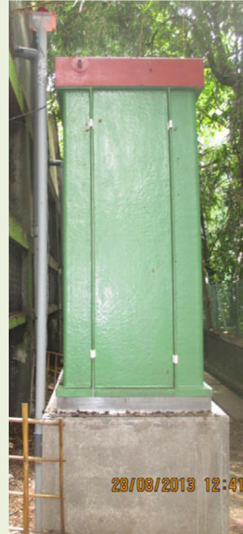
Vent pipe for solids pit
