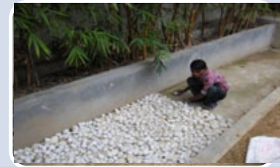
Planted Gravel Filter Bed (Secondary and Tertiary)
