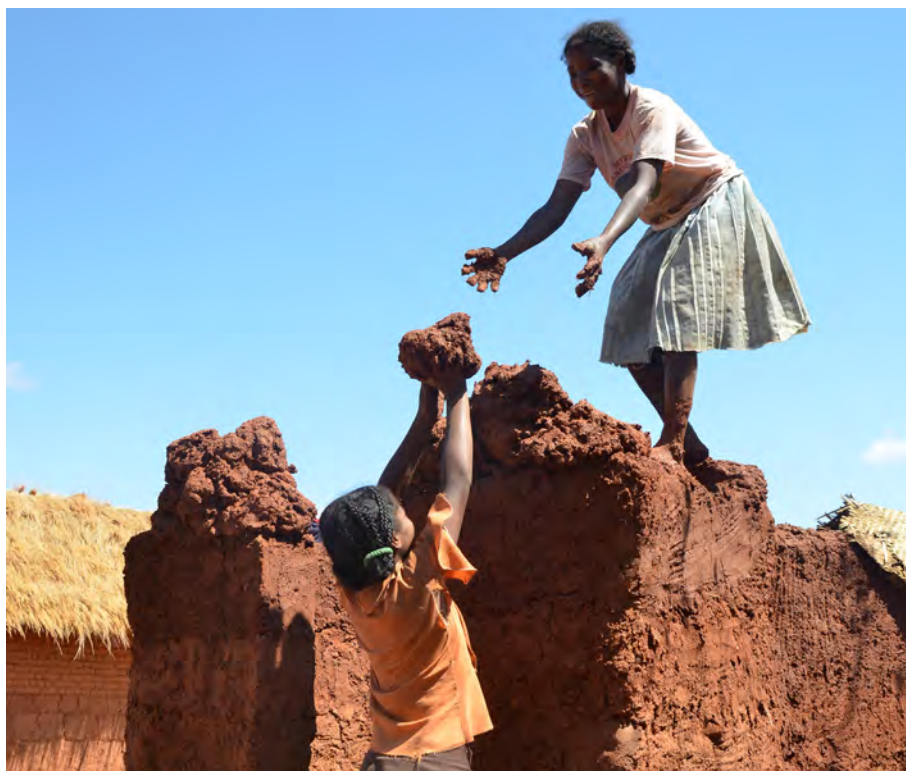
Zinah and her daughter, Zin, 13 years old, building their toilet. Ambohimasina village, Talatan' Angavo commune, Ankazobe district, Analamanga region, Madagascar, October 2013. Credit: WaterAid/ Ernest Randriarimalala.
