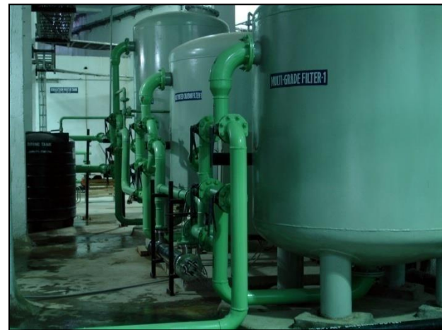
Overview of the Tertiary Treatment
