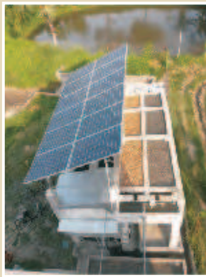
Top view on HRF/SSF/ACF filters with PV cover
