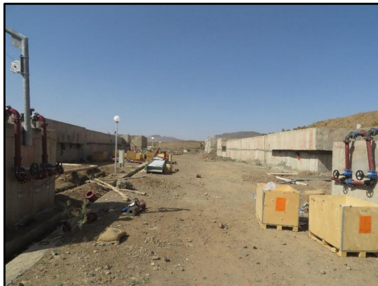
Figure 7: New wastewater treatment plant under construction in Axum University (photo credit: Oscar Veses).
