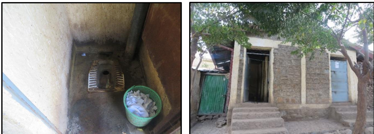
Figure 3: Inside and outside of a public latrine (photo credit: Oscar Veses).
