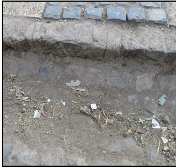
Figure 6: Drainage system (photo credit: Oscar Veses).
