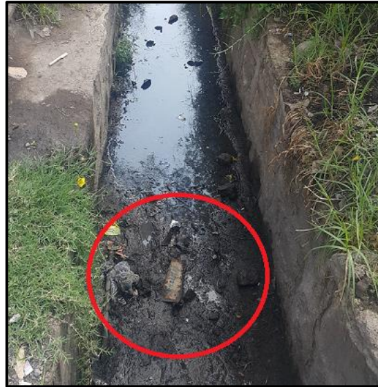
Figure 8: Drainage system (photo credit: Haile Dinku).
