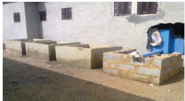
Primary treatment pit
