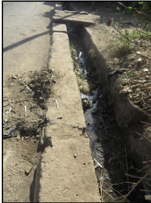
Figure 13: Drainage system (photo credit: Oscar Veses).
