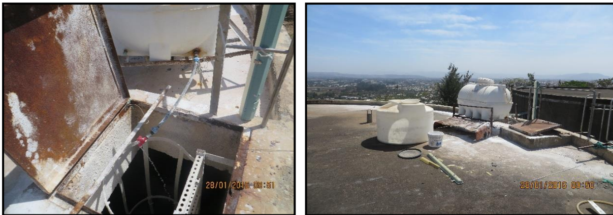
Figure 15: a) Chlorine manual dosing tank. b) Storage reservoir for Tiqurwuha, Lome and Areki springs (photo credit: Eshetu Assefa).
