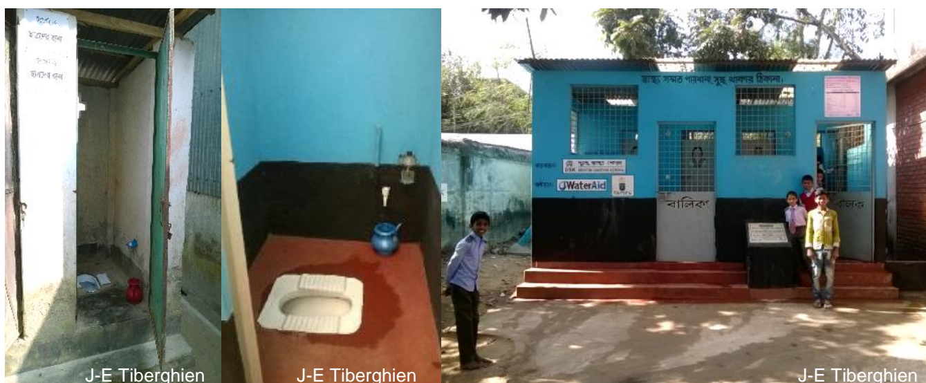
Old yet well maintained and functional toilets in Jamila Akter high school, Fulchari, Gaibandha (left). Brand new, gender-separated WASH block built in IPH school and college, Mohakhali, Dhaka (middle and right).
