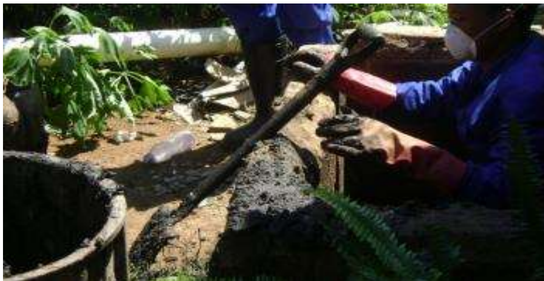
Figure 23: The lip of the pit typically became heavily soiled during emptying
