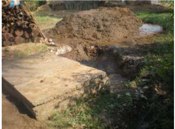
Photo 3 Outlet chamber with slurry tank being cleaned recently
