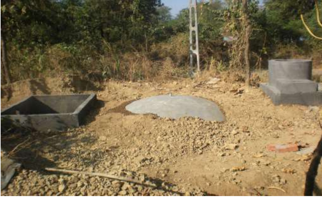
Photo 11 Almost complete biogas plant only outlet chamber is to be covered with slabs
