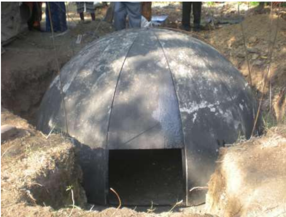
Photo 8 Steel mold of biogas plant put for completing upper part of the plant
