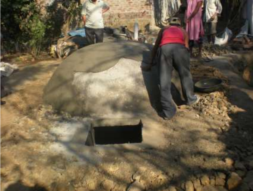
Photo 9 Biogas plant with completed dome. Inlet tank and Outlet chamber under construction.
