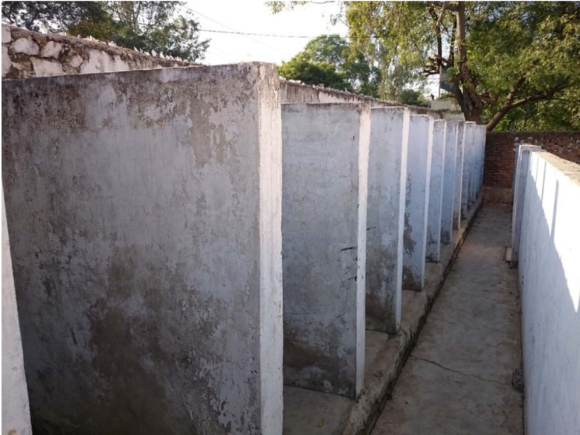
Many urinals, but their quality is poor and urine flows into a drain outside. Pic: Nitya Jacob
