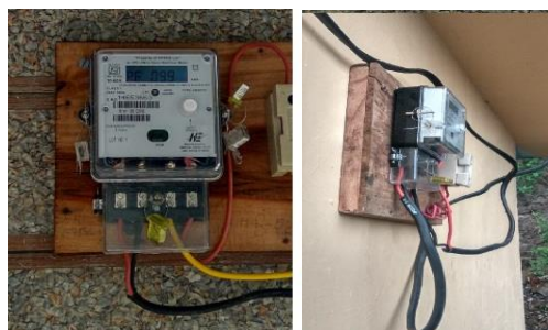
Pic: Electricity Meter exposed @ Ram Mandir Public toilet, Shimla
