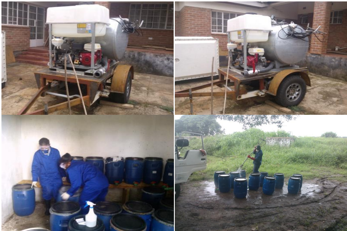
Figure 3.5 ROM2 Desludging machine & 50 litre fermentation reactors
