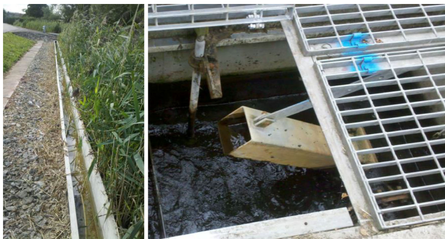
Figure 3.2 Examples of civil structures in HF wetlands; left: distribution troughs; right: water level control structure.
