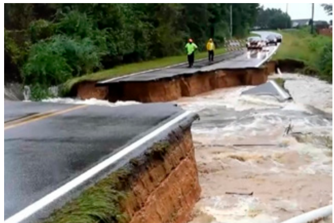
The destruction of the East-West Highway during the 2014 flood tragedy
