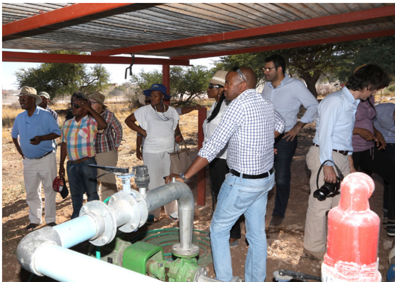
Borehole for irrigation in the Stampriet Transboundary Aquifer System
