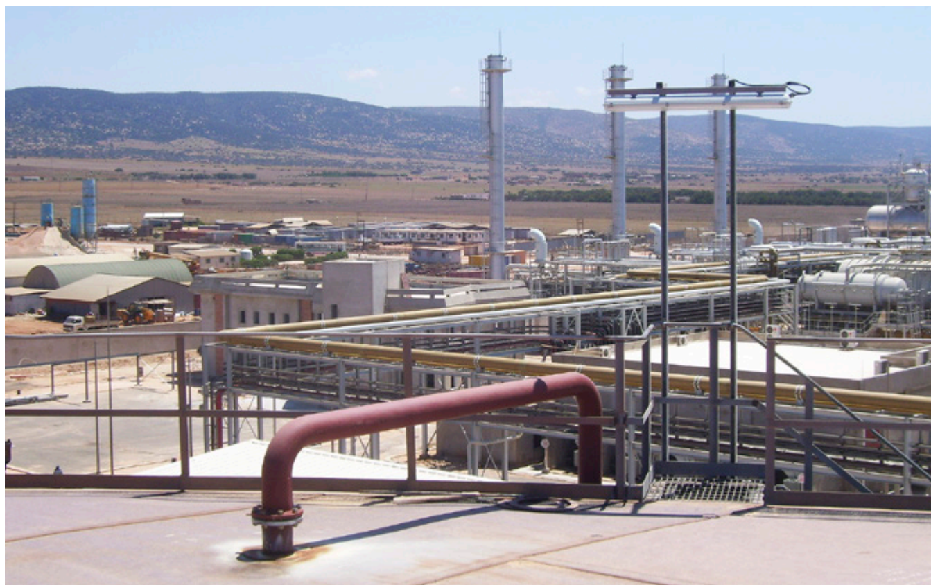
The 40,000m 3 /day Butraba desalination plant, constructed in 2007 for domestic water supply to Al Marj city and surrounding urban areas in north-east Libya
