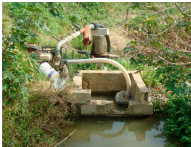
Uncontrolled and unmaintained boreholes are common in Lebanon
