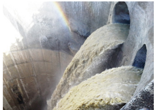
Sarabium siphon, 60m below ground, built to transfer agricultural drainage water to the eastern part of the Nile Delta
