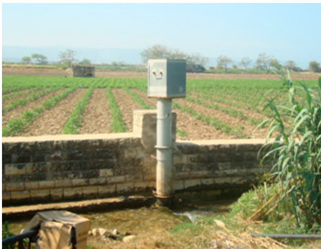
An old and unmaintained flow-meter
