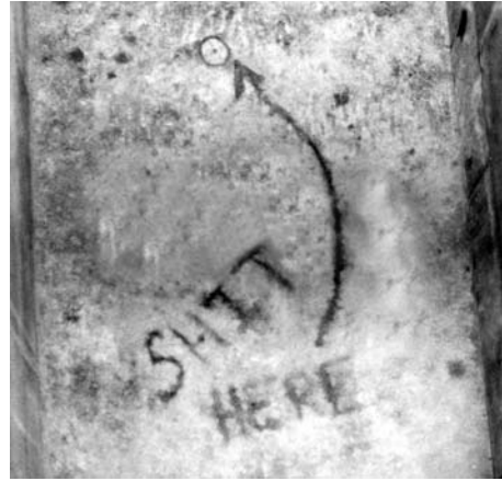
NEW, OWNER-BUILT COMPOSTING TOILET CONCRETE FLOOR with engraved instructions for use
