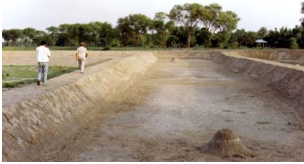
Photograph 24: Duckweed-based sewage treatment lagoon of PRISM Bangladesh at Mirzapur showing one reach of the plug-flow channel under construction. (Photograph: PRISM).
