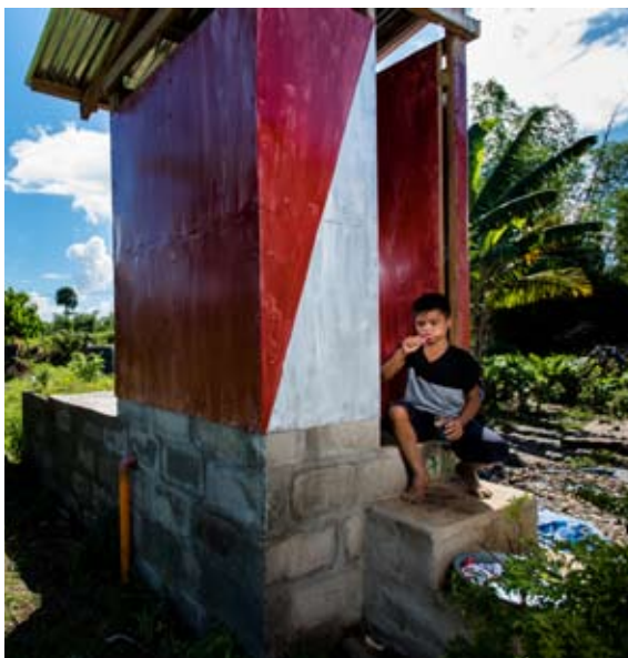
Below: The Type 7 toilet and septic tank is for households whose groundwater level is between 0.65 and 1.5 meters from the natural ground.
