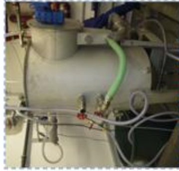
3 - Pretreatment tank Volume of tank: ~ 400 l
