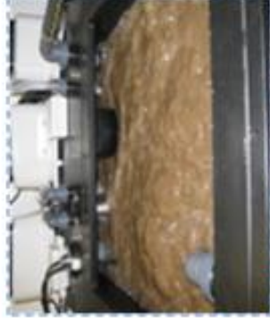
4 - Membrane bioreactor Volume of tank: 710 l
