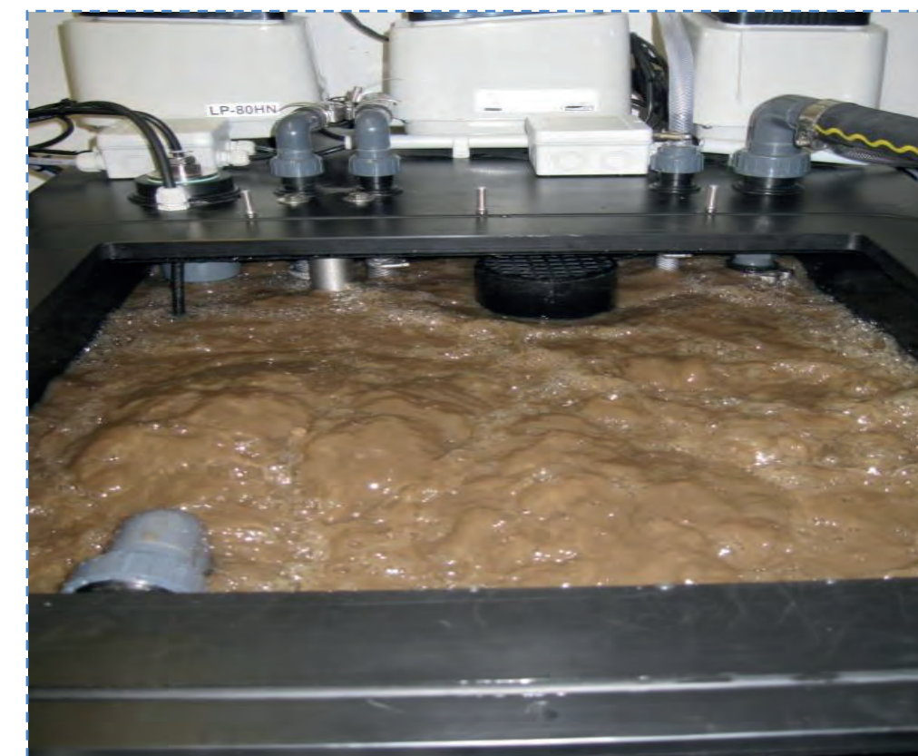
4 - Membrane bioreactor Volume of tank: 710 l
