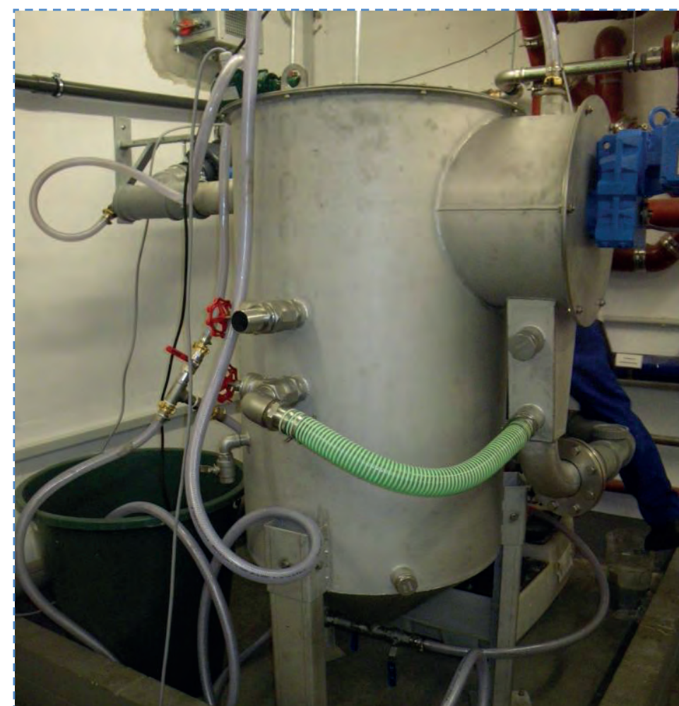
3 - Pretreatment tank Volume of tank: ~ 400 l
