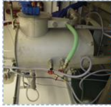
3 - Pretreatment tank Volume of tank: ~ 400 l
