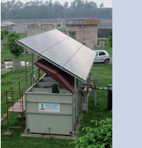
Demonstration system at the Yamuna Vihar treatment plant in New Delhi, India
