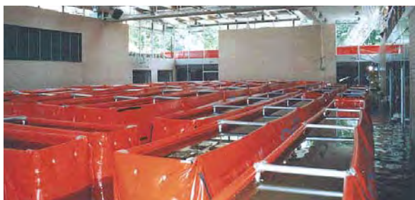
Protecting the building structure against rising groundwater at a Dresden school (Source: www.benno-gym.de)
