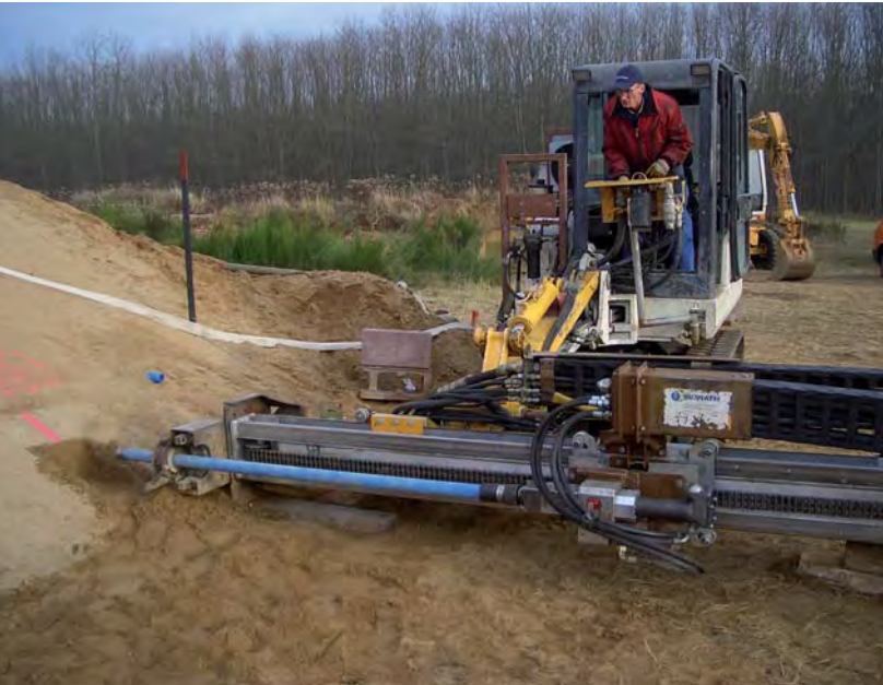
Standard drilling is to be applied to implement the linear drainage elements in the model dyke (Performed by: Morath GmbH, Albruck)
