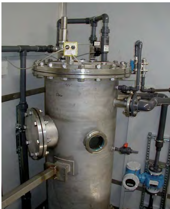
Reactor for biological nitrate removal (denitrification)
