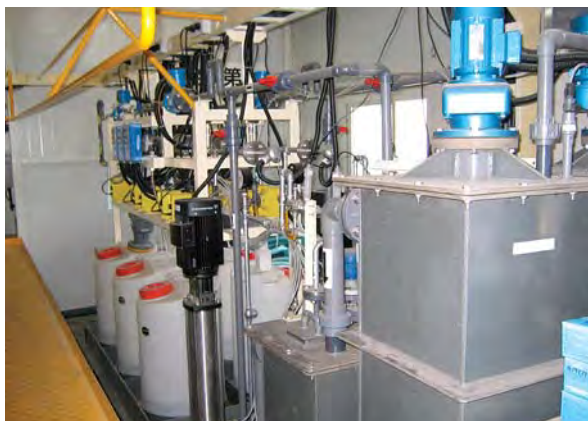
Part of the pilot system at the BeiXiaoHe purification plant
