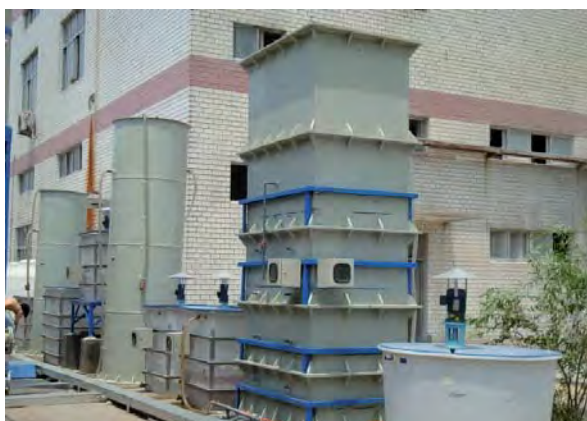
Iron bed (foreground), intermediate treatment and final clarification (background)
