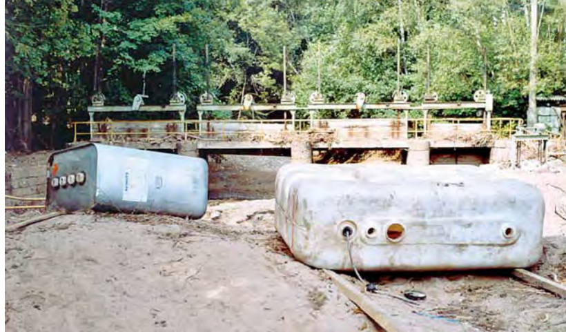
Oil tank torn off by the Elbe flood (Source: Thomas Egli)
