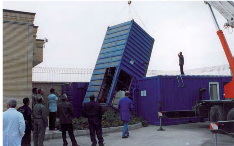
Erection of test systems on the grounds of the well pump station in Mashhad
