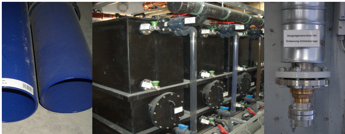
Figure 4 Pipes of cast iron with enamel coating (left), urine tanks (middle), and docking station for tank trucks (right) (source: GTZ)
