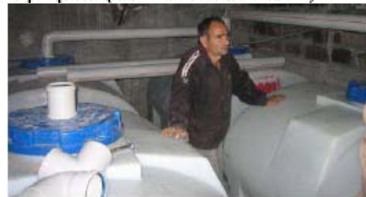
Figure 10: four urine tanks are deposited in the basement of the school (source AWHHE)
