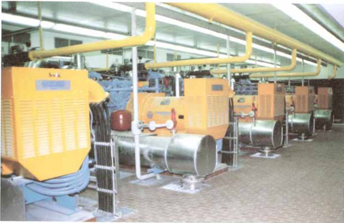
Block heating power station
