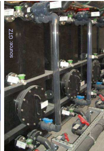
urine storage tanks (4 x 2500 L)
