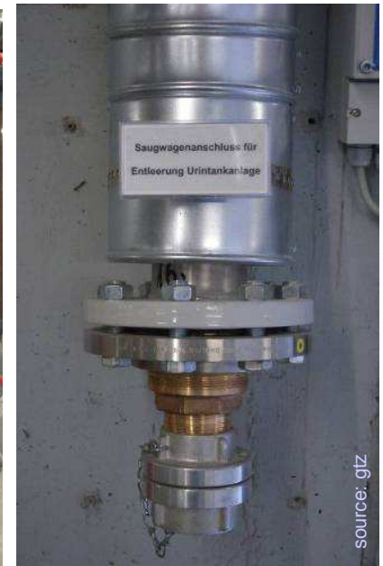
docking station for vacuum tanker
