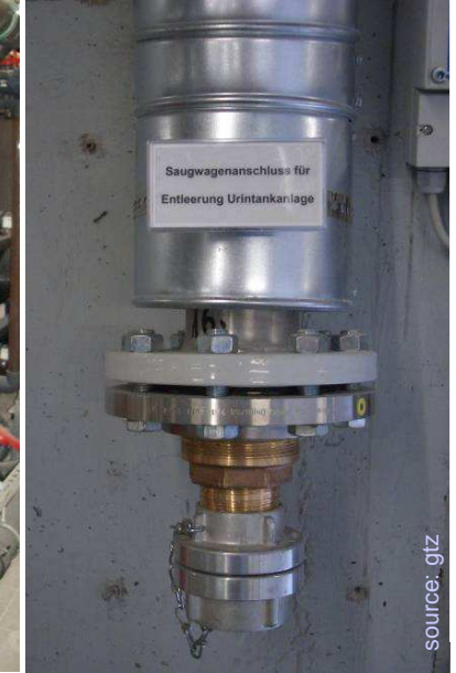
docking station for tank trucks
