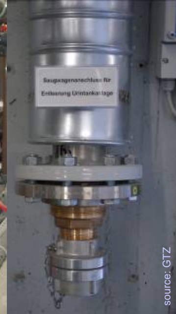
docking station for tank trucks
