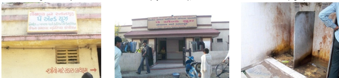
Figure 10 Pay & Use Toilets in Ghatlodia (left & centre); Urinal without water connection (right)
