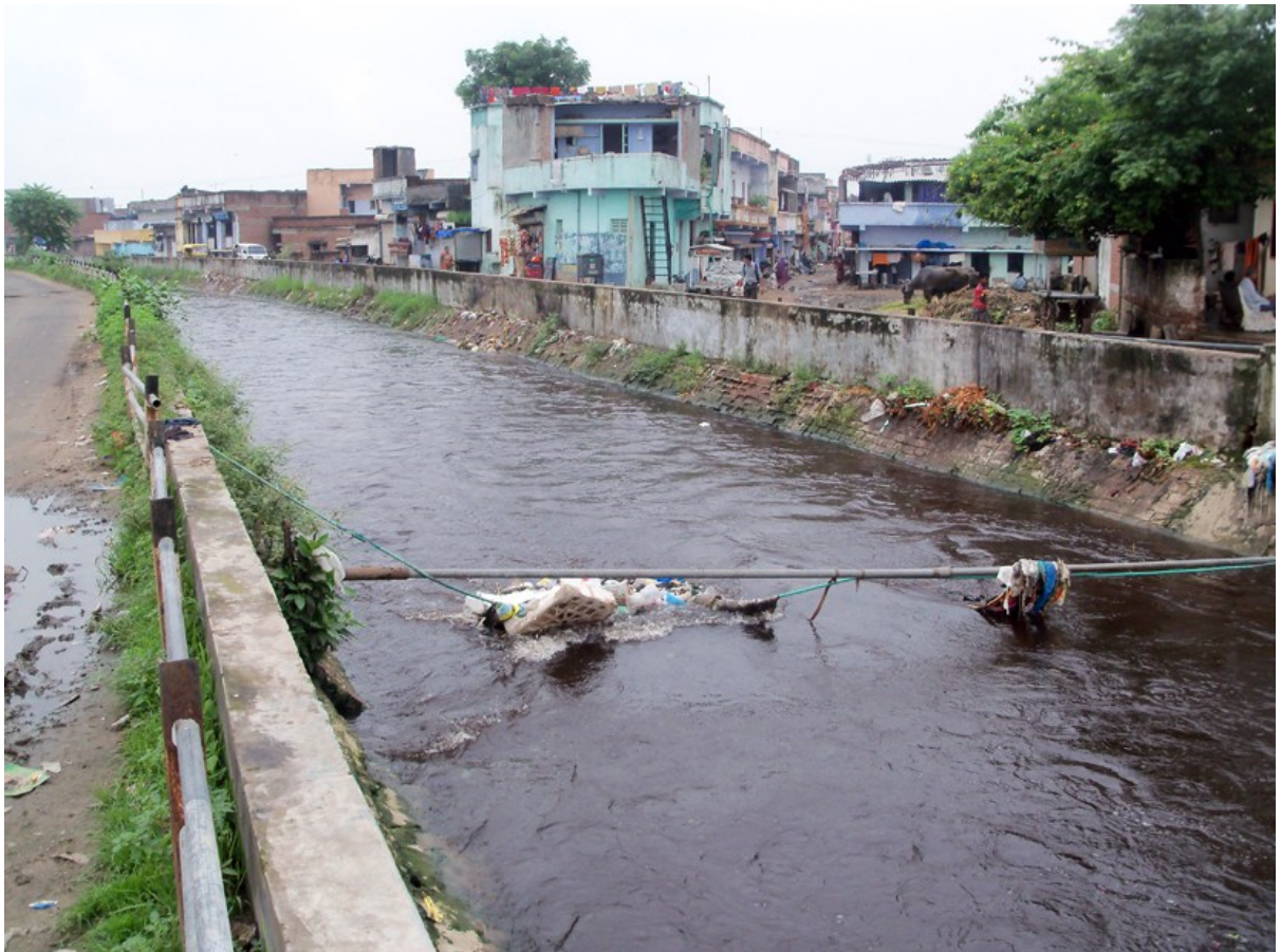
Figure 18 Khari Cut Canal - facing the brunt of solid waste, sewage and industrial effluent disposal
