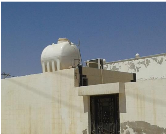
Rooftop water tank in Za'tari village
