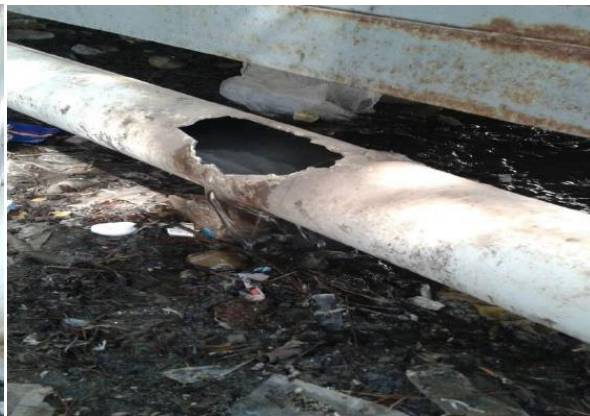
Sewage pipe in the Sport City Center that shelters refugees
