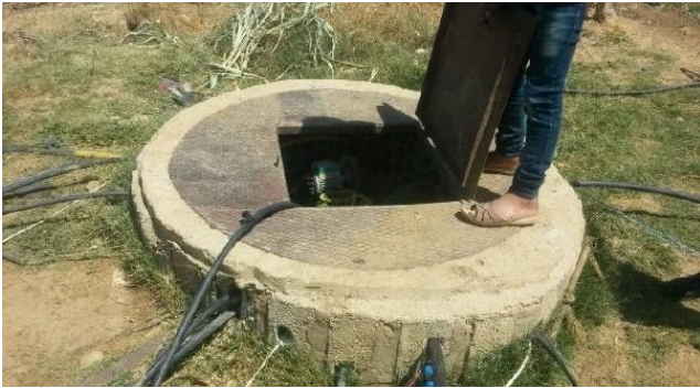
Artesian well pumping water to Hosh Rafqa peoples' house tanks
