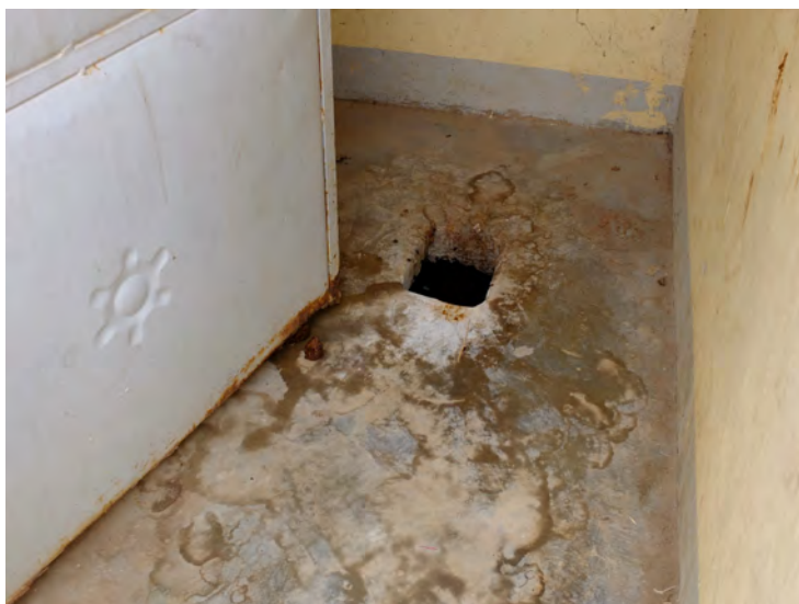
Latrine inside 5 stance VIP latrine at School 2, February 2017
